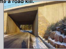
Fig. 5: Underpass with county road: dangerous crossing possibility
